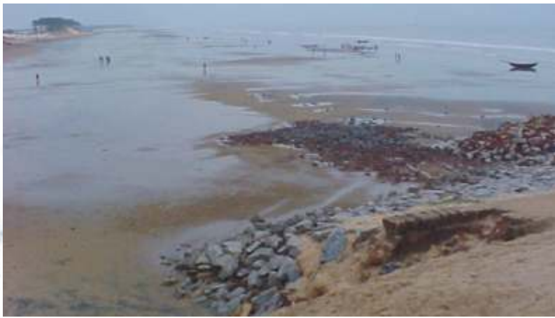
Fig. 11: Rolling of Boulders of the sea wall at Digha due to wave action
