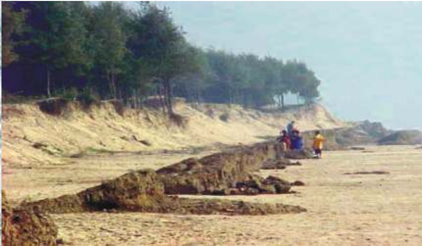
Fig. 13 Exposed and eroded Earthen Embankment of Shankarpur
